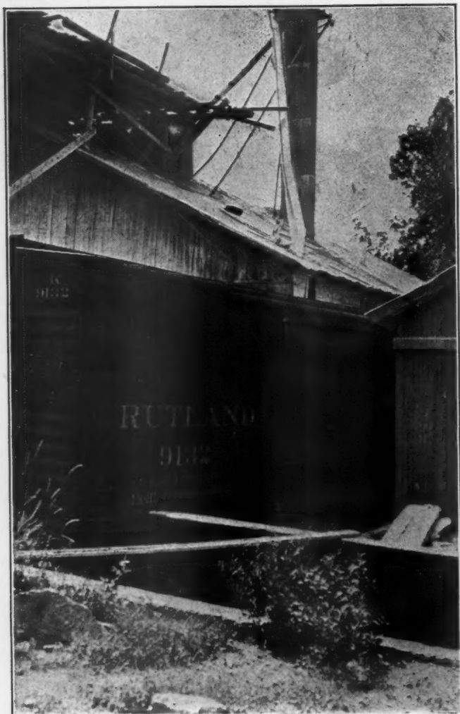
Top of Elevator Associated with Hammer Mill Showing Chutes Extending to Storage Bin
